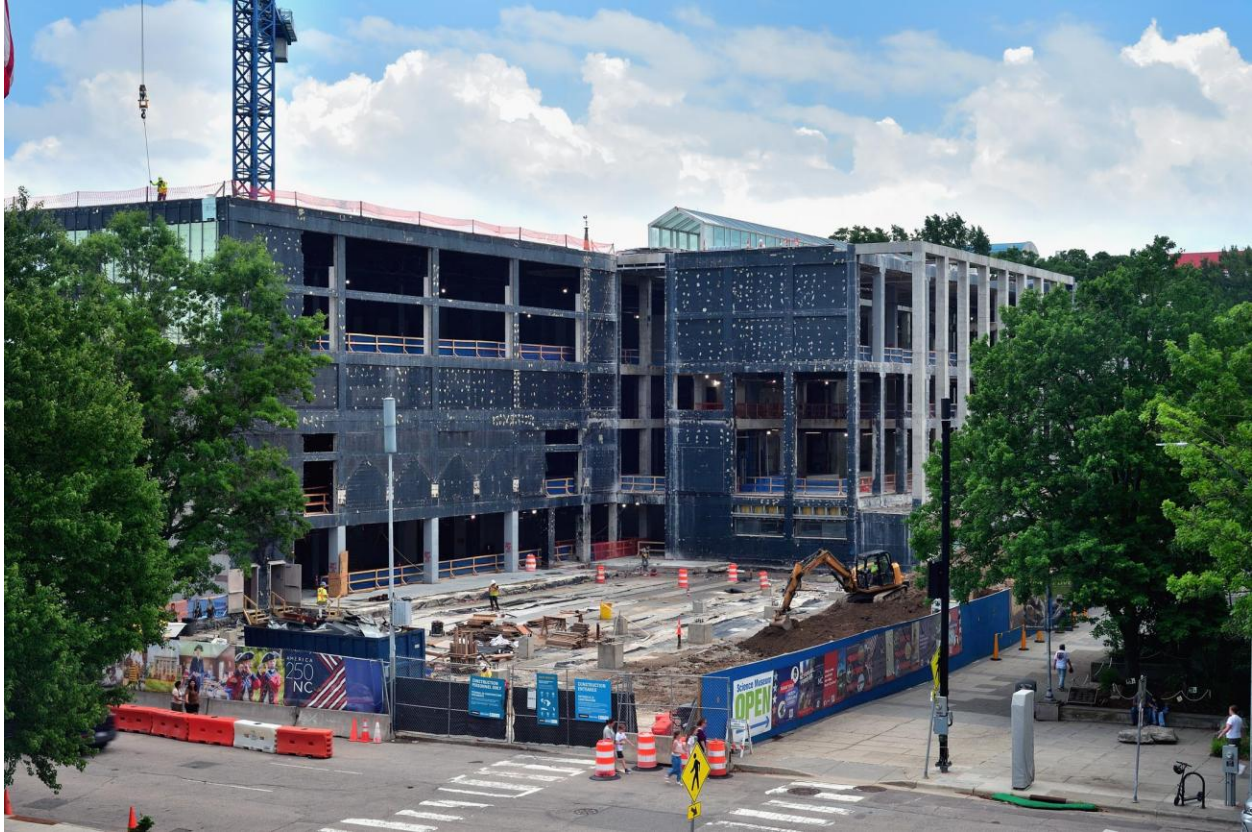
Figure 3: View of the northwest corner of the NCMOH building from June 2026. This will be the location of the new lobby.
