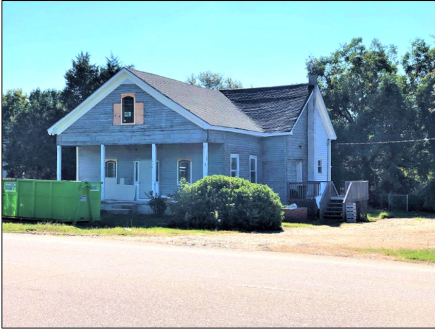
Photograph 21: Former house of worship, view southeast. Note window modifications.
