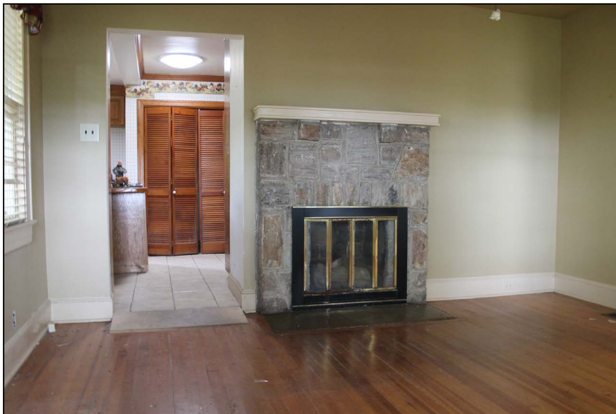
Figure 4.17: Joseph Collier house, view through broken window into rear of original house, facing north.
