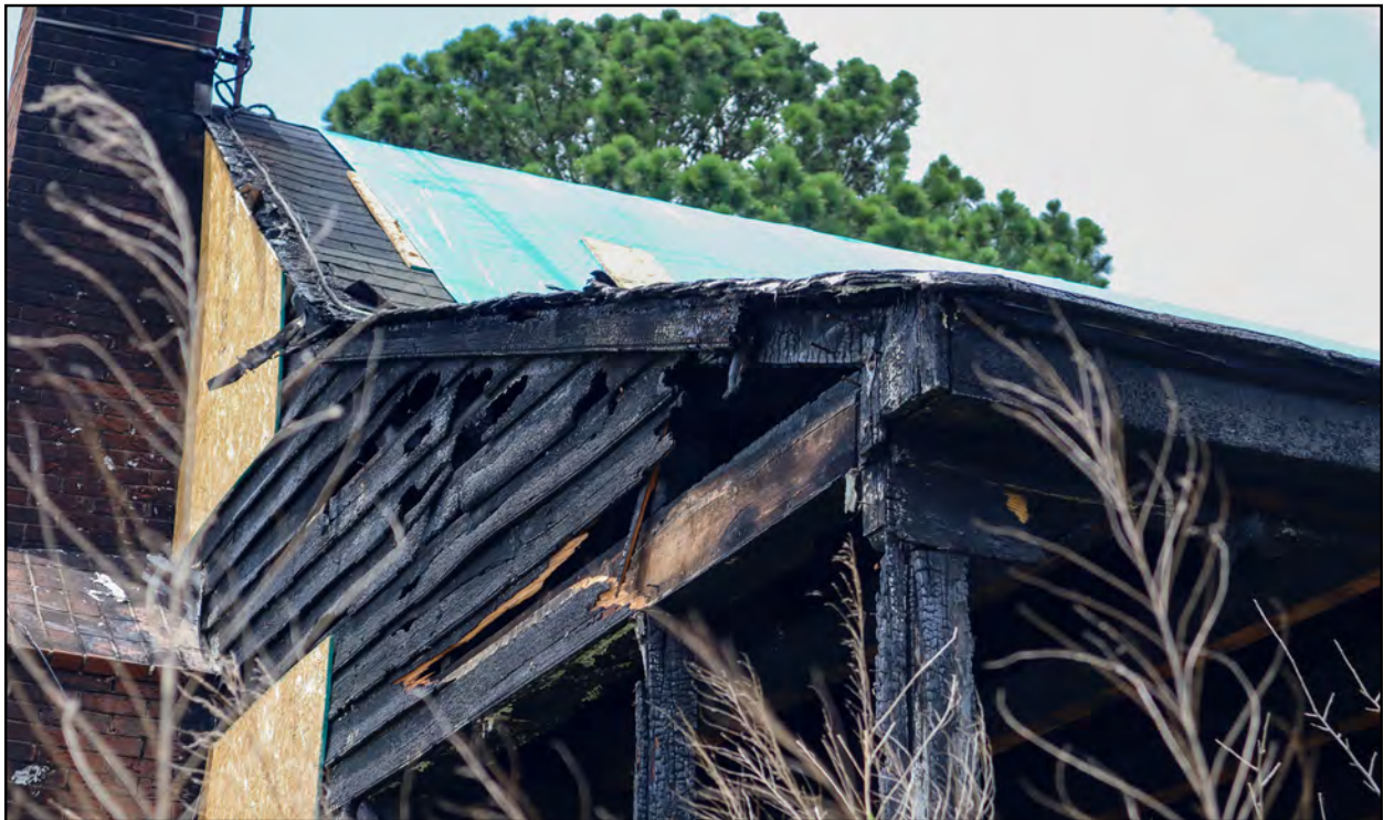
Figure 4.17: Detail view of the original beaded weatherboards on the south elevation that were damaged by the fire.
