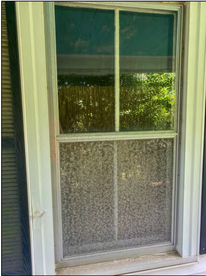
Figure 4.16: Detail view of an intact, original window in the I-house section of the Hunter-Prince House
