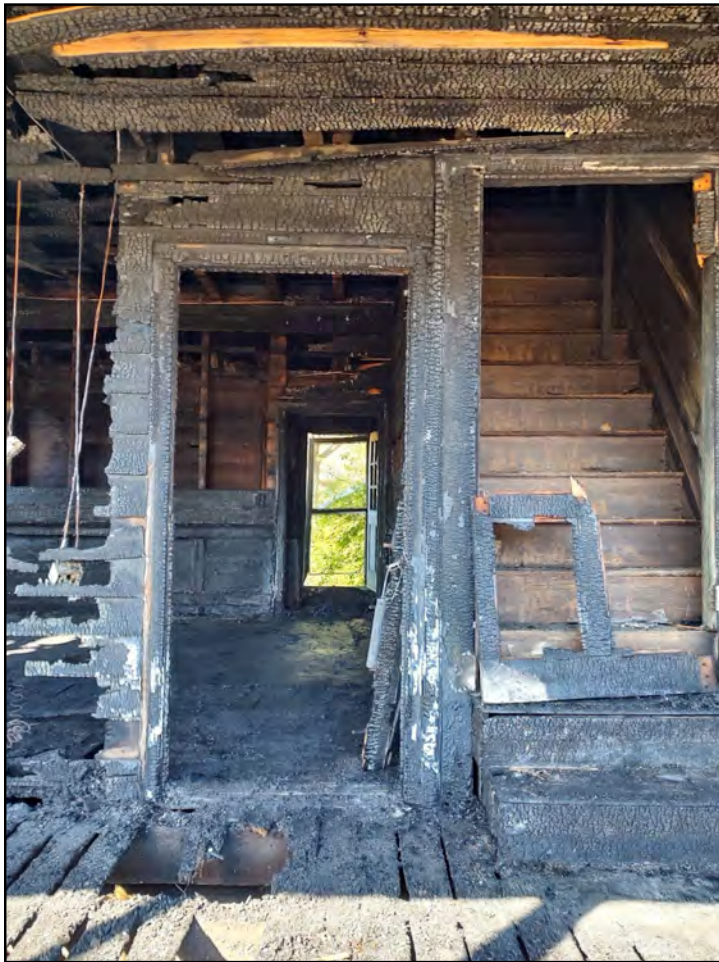
Figure 4.20: View of the circa-1810 section of the Hunter-Prince House shortly after the fire in April 2022. The view looks through the front door and into the hall of the house. Note the exterior stair to the left of the front door (Courtesy of Jeremy Bradham, Capital Area Preservation)..
