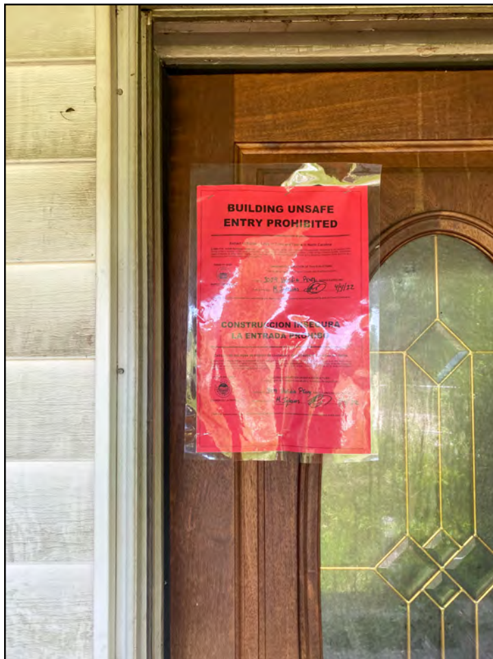
Figure 4.14: Entry prohibited sign from the Town of Apex on the front door of the Hunter-Prince House.
