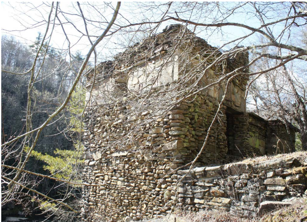
Plate 3.2: Powerhouse on the north end of Sloops Lake Dam (AV0082).
