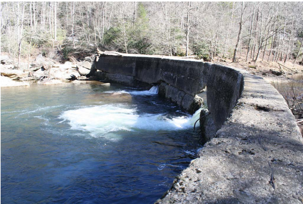
Plate 2.3: Shulls Mill Dam.
