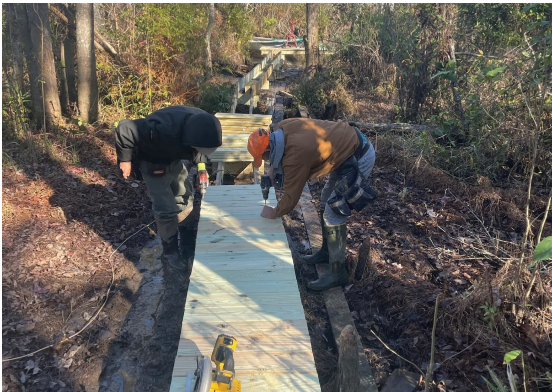
A Complete the Trails Program project in progress at Cypress Cathedral on the Roanoke River State Trail
