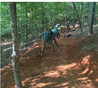
CCNC crews construct connector trails to the new Eno River State Park visitor center
