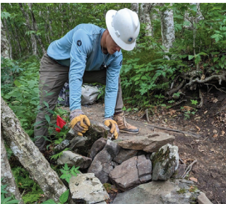
CCNC Crew member repairing rock work on the Summit Trail at Elk Knob State Park
