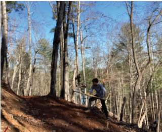
CCNC/NC Parks Trail Technician Arey Clark building new trail at Lake James State Park
