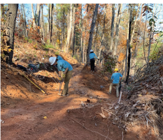
CCNC Crews build a trail from the newly constructed Visitor's Center at Lake James State Park
